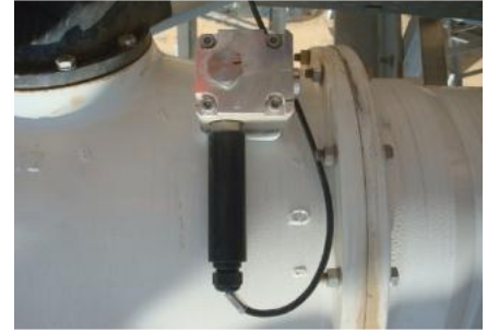
Gas sensor - Outdoor (sun, rain protection)
