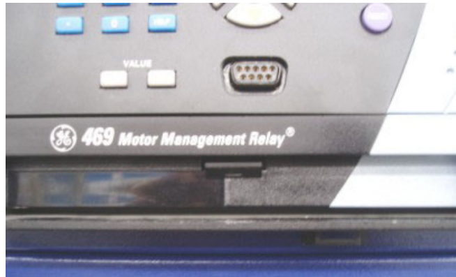
FIGURE 3-2: Seal on Drawout Unit
